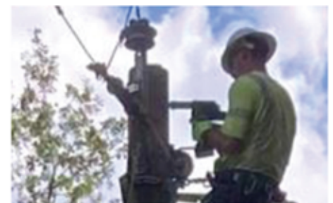
Steele-Waseca Line Technician Carlos Cruz works on hanging new wire to a pole as part of the effort to restore power in South Carolina following Hurricane Helene.
