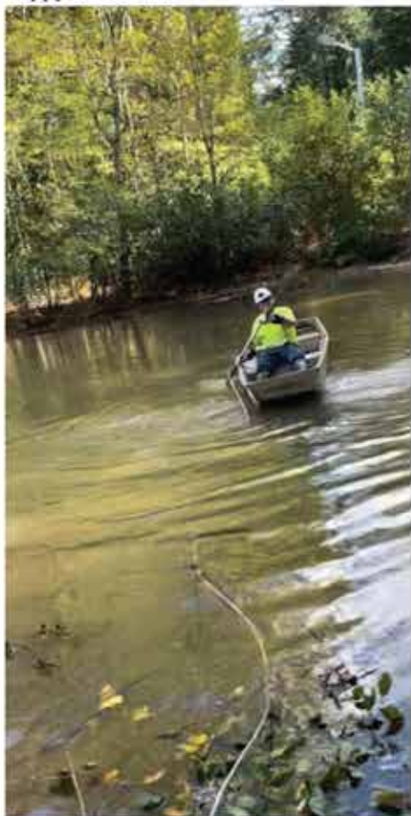
Assistant Foreman Jake Jablonski needed to utilize a boat to transport line to a power pole in South Carolina.
