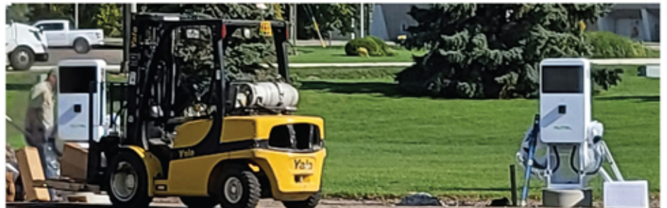
Steele-Waseca Cooperative Electric Master Electrician Joel Dulas (pictured far left, obstructed) conducts electrical work, Oct. 2, for the chargers prior to transformer installation.
